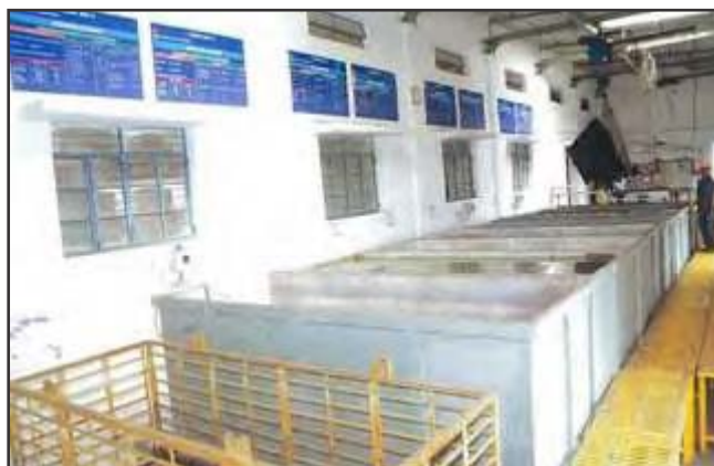
Powder coating unit at Dharwad
