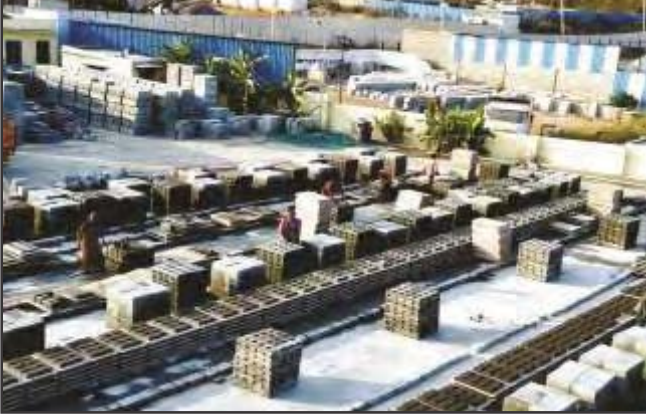
PCC hollow blocks Manufacturing unit at Bengaluru
