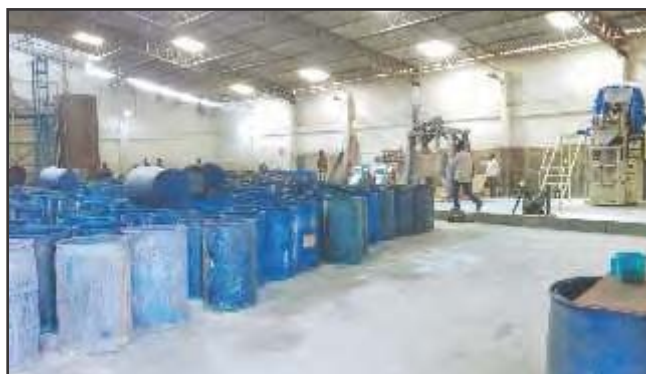
Chemical unit at Hassan
