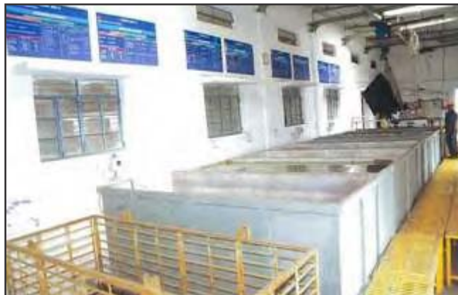
Powder coating unit at Dharwad
