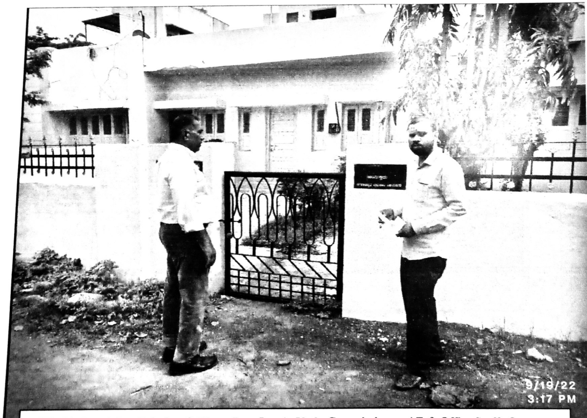
S.L-31 Repairing, Painting & Water Proofing At Vuda Commissioner, AE & Office Staffs Quarters.
